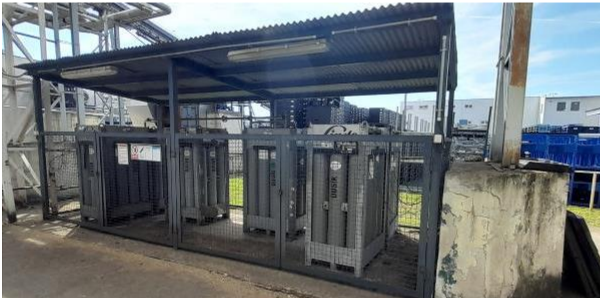
Fig. Detail of the connection of the nitrogen pressure cylinders
